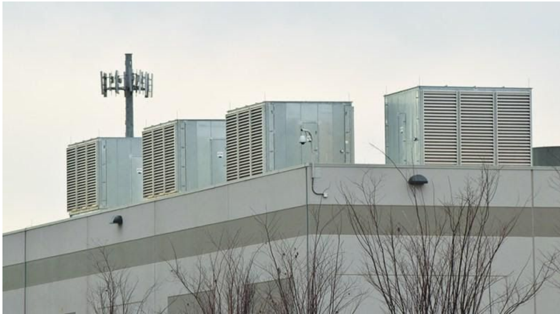
Image of early data center (Courtesy Loudoun Now)
